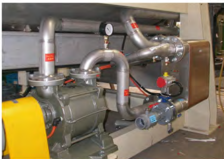
Drying & Cooling System
